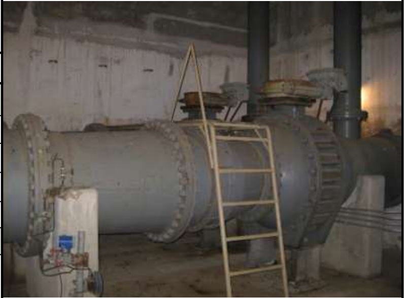
Pictured above: Ball valves located in the Right-End Pier Low Flow Facility
