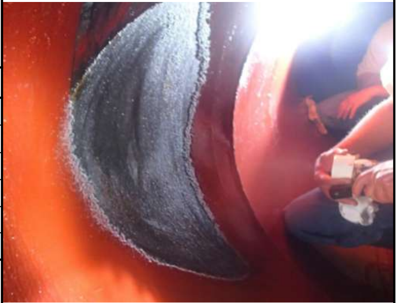
Pictured above: Coating eroded from pipe wall
